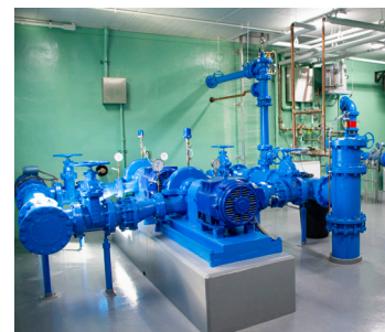
Well No. 6 Pumping Station
